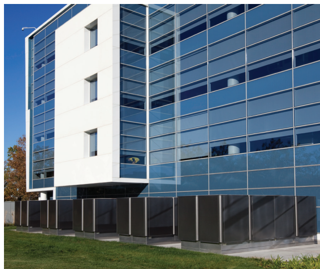
FIGURE 6: Bloom Energy Server Outdoor Installation
